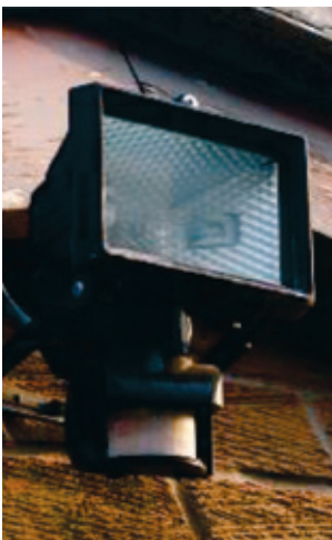
Event activated lighting is a familiar feature
